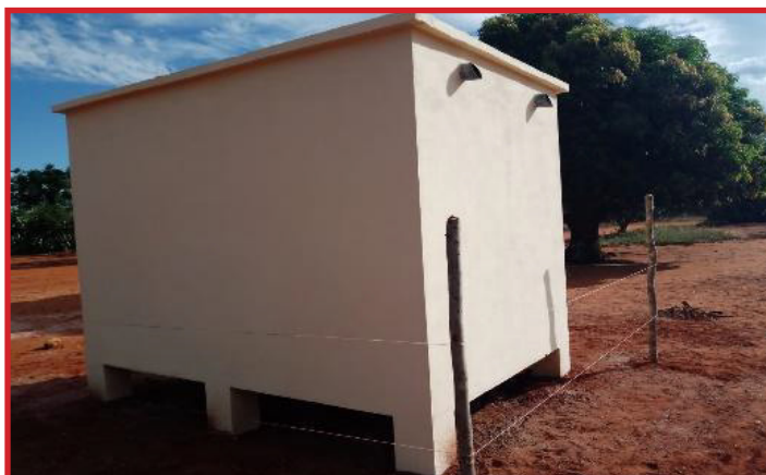
A newly installed water tank
